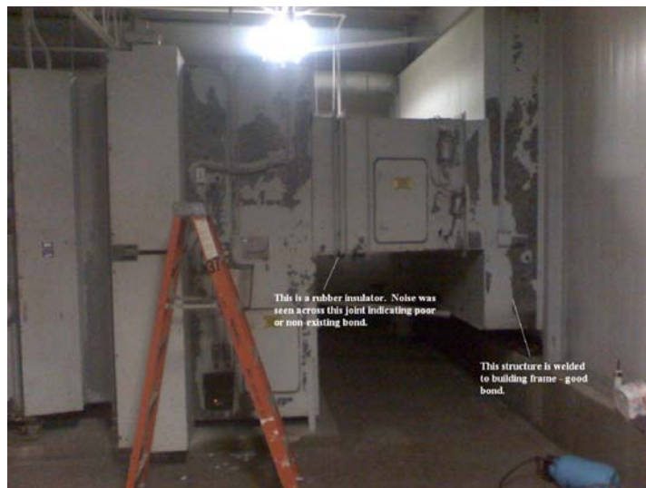
This is the part of the air handler closest to the building structure.
