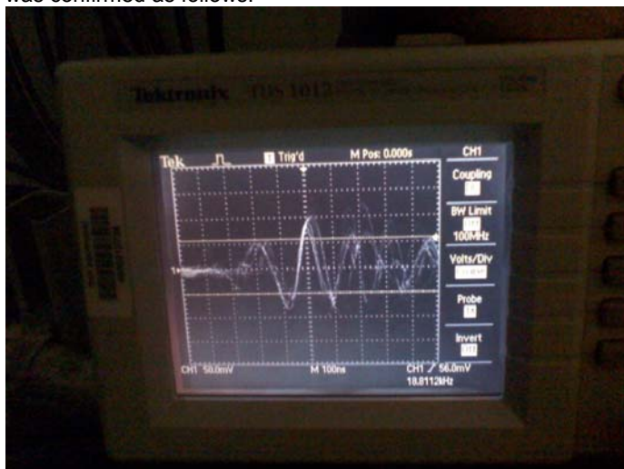
This is the waveform that was found at various places on the air handler.
